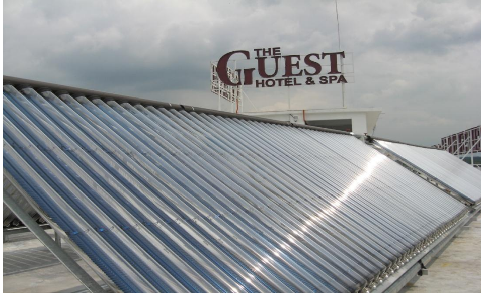
Heat pipe vacuum tubes of the Guest Hotel
