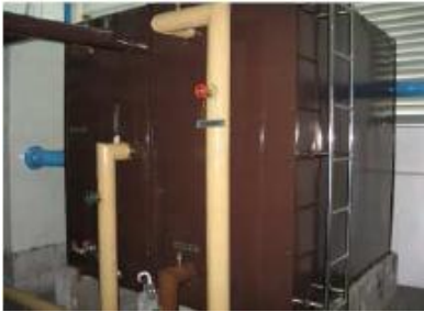
Hot Water Tank
