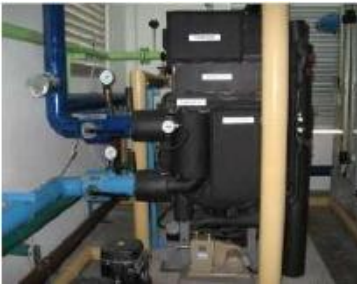
SDC Absorption chiller
