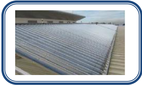
SDC Solar Collectors
